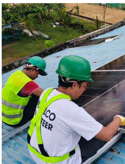
Solar panels were installed to power Homonhon Island Community Hospital, allowing health workers to serve patients anytime.
