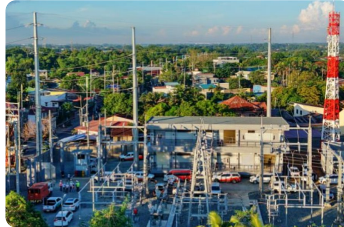
Development of Bustos 69 kV-13.8 KV Substation
