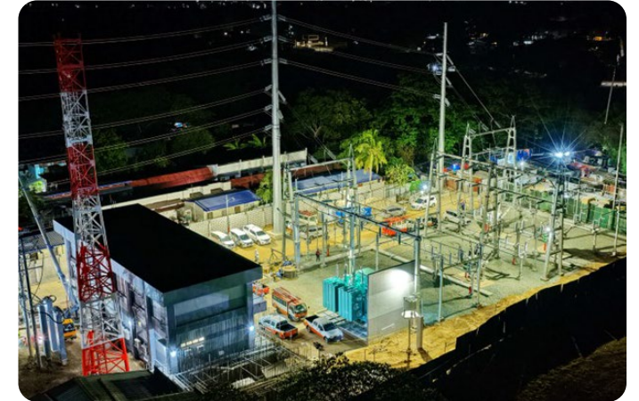
Development of Osorio 115 kV-34.5 kV Substation
