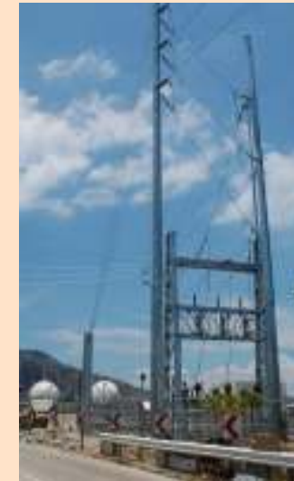
JG Summit's Metering Facilities
