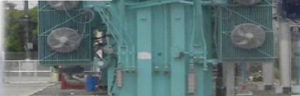
Expansion of Dolores Substation (2nd Bk)
